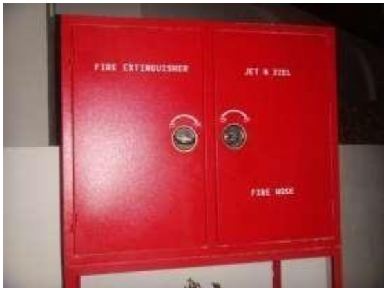
HOSE REEL CABINET
